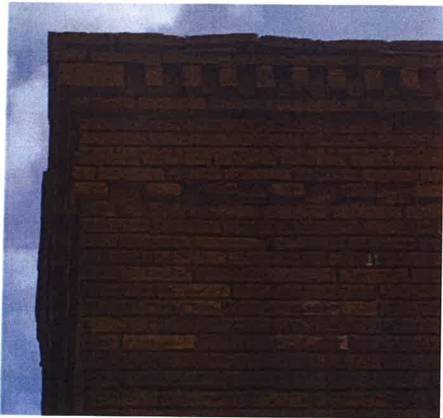
Loose and missing bricks along the parapet of the building.
