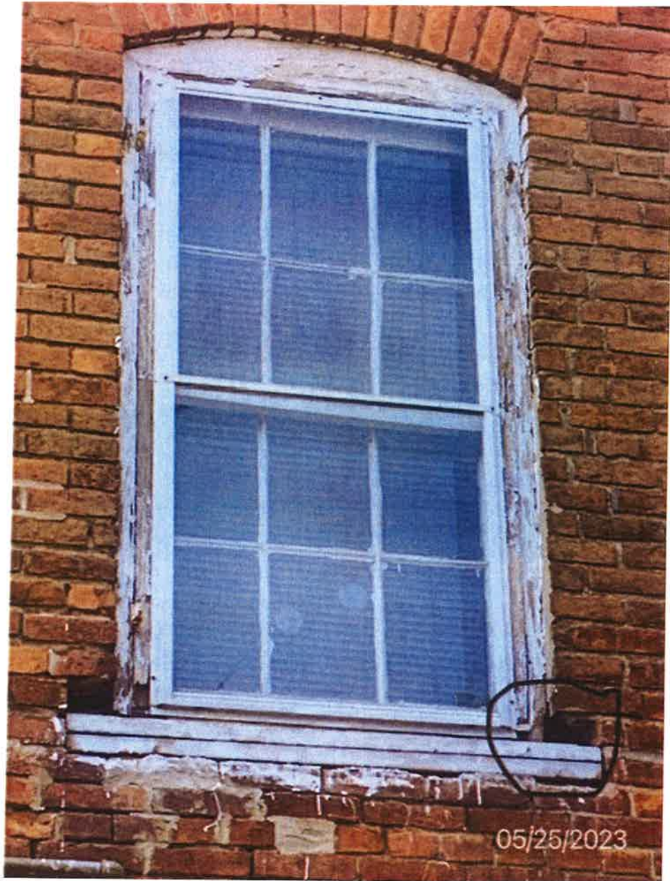
Same window as previous photo. Brick in lower right hand corner now missing – May 2023
